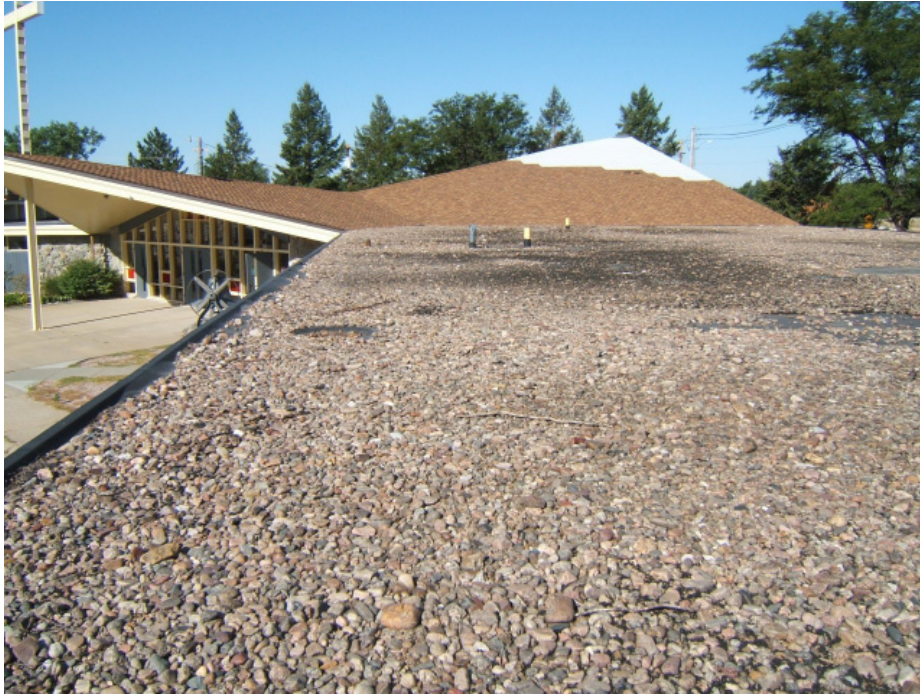
Roof damage to Valentine Presbyterian Church.
