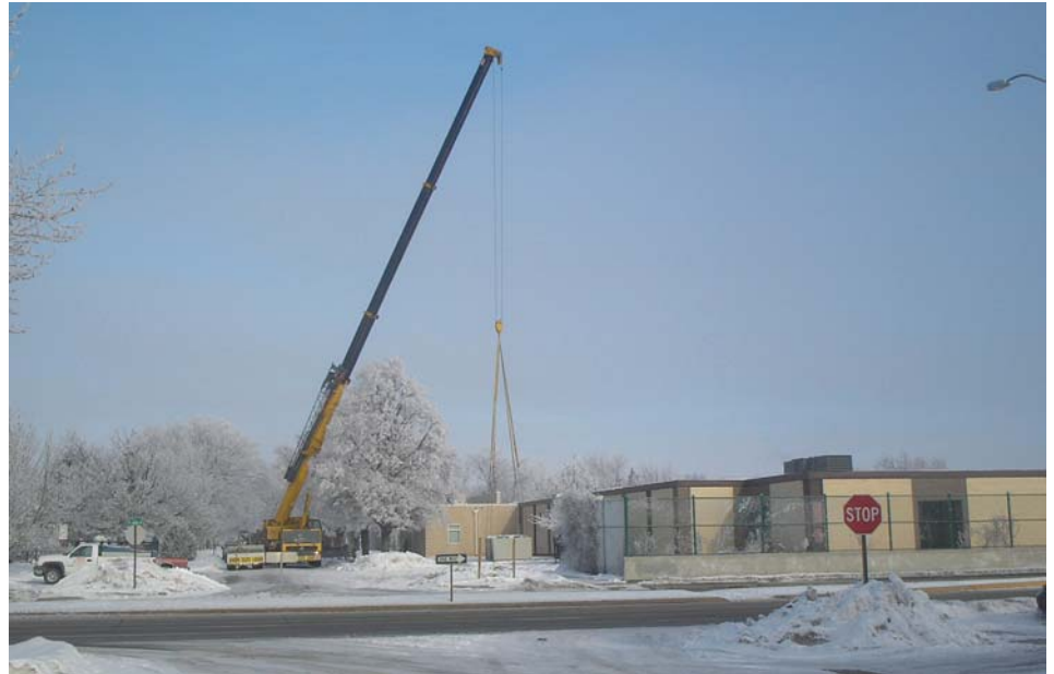
A crane prepares to set the new air handler on the roof at Washington Elementary.
